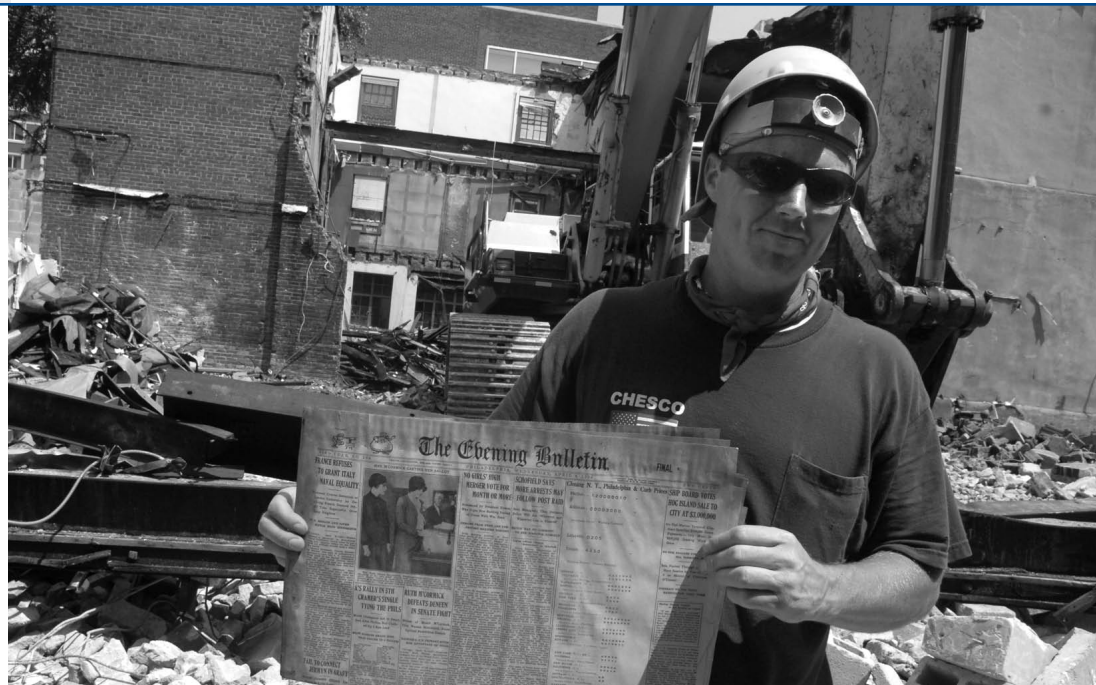
A construction worker displays a copy of the Philadelphia Evening Bulletin from the 1930s, which was unearthed during demolition of the Hillel House. Demolition is the first step toward construction of the new Annenberg Public Policy Center.
